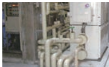
Bathroom heating system with filtration unit
